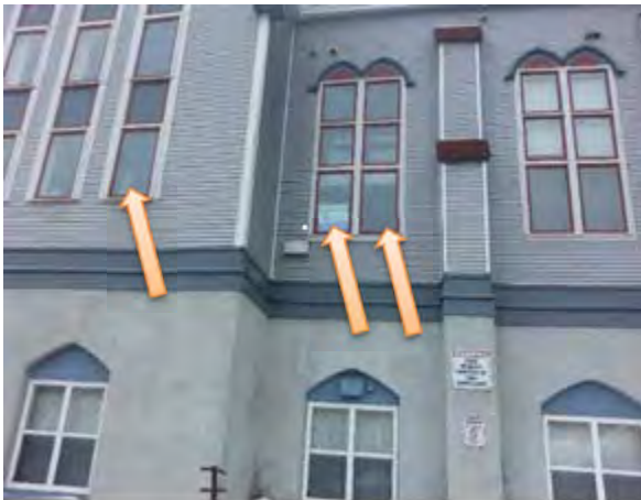
Windows to be Replaced
