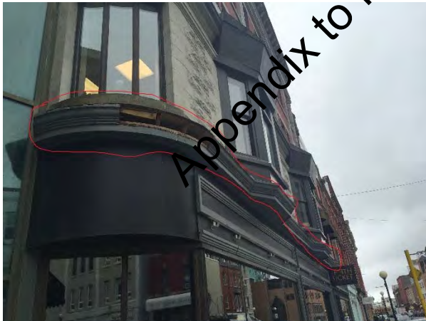
Area of moulding to be replaced Colour to match - Dark Grey
